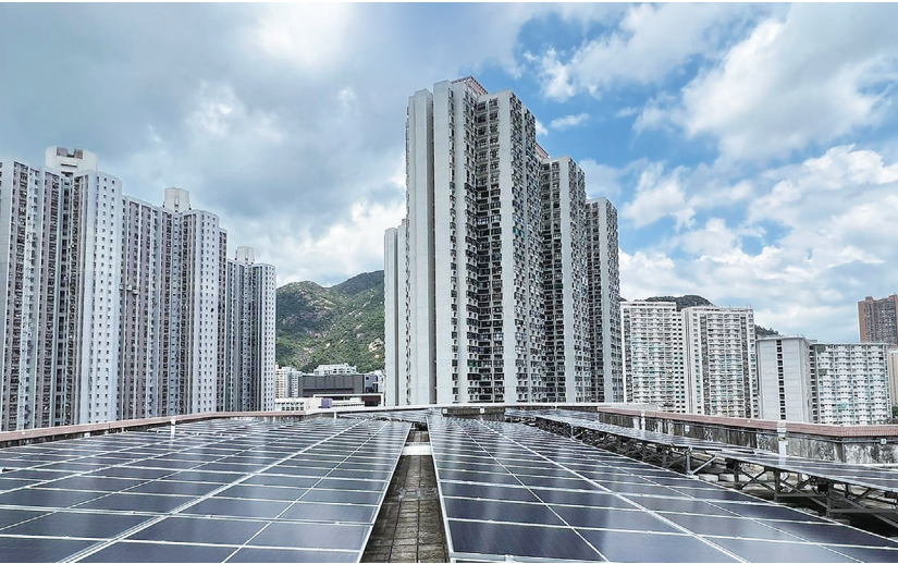
PV panels installed at HPML managed assets
